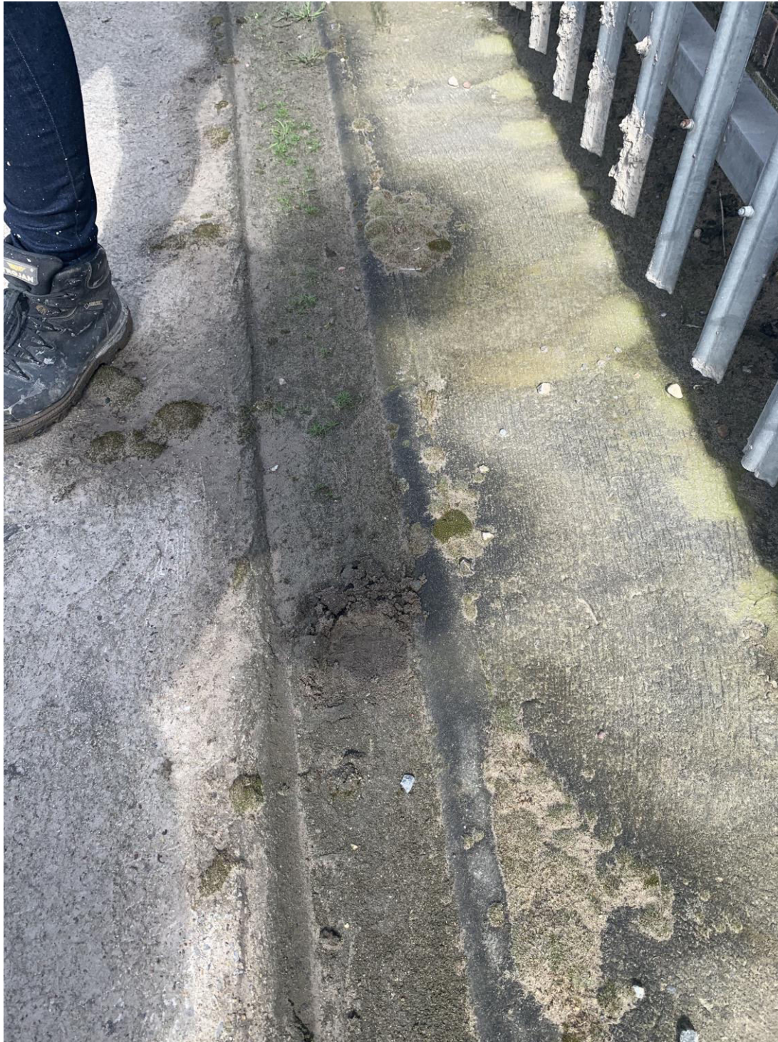
Photo 4: Dust accumulation in pavement drainage gully.
